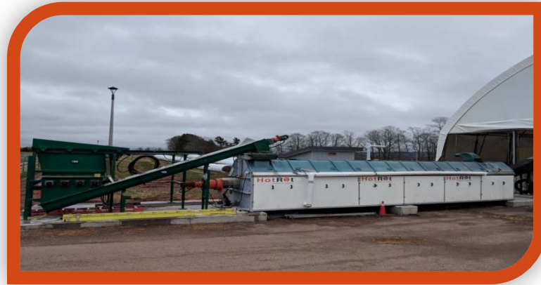
Fig. 1. HotRot 1811 composting system located at Dalhousie University, Nova Scotia, Canada.
