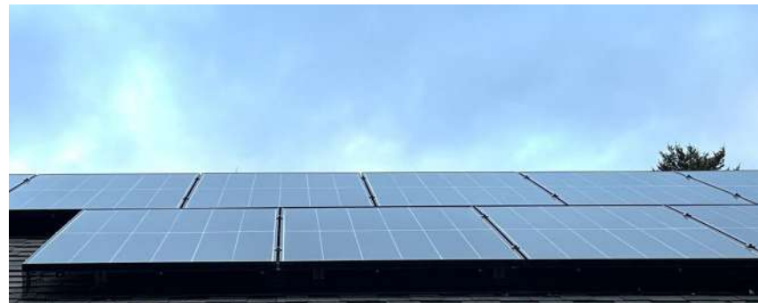
Wire mesh guards below the panels
