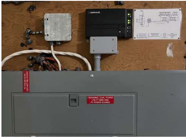
In house meter
